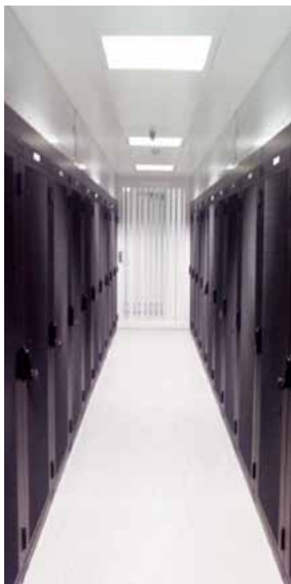
Rack space in Merlin
