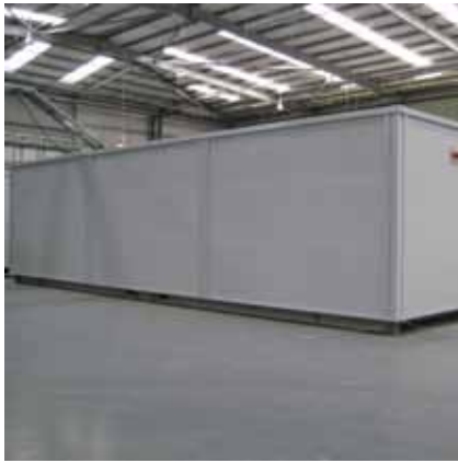
Data centres traditionally carry an extremely high capital cost, and depreciation starts from the first day of production
